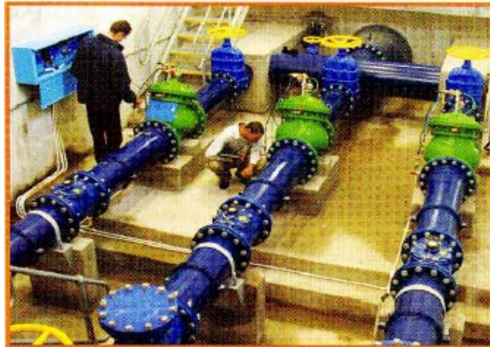
Figure 3: Khayelitsha township pressure management system with BERMAD pressure reducing valves.
