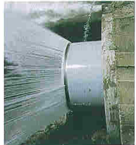
A 54-inch Hartman Fixed Cone Valve operating in the almost closed position, discharging 1 cfs. Note the fully circular flow.
