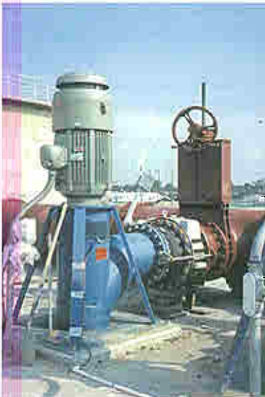
30" Flexgate Valve at the Donora, PA WWTP
