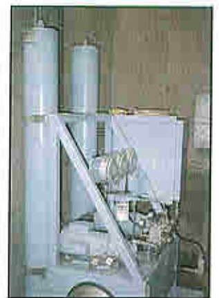
Oil hydraulic power package with back-up nitrogen accumulators.
