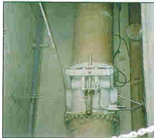
This valve has a 36 inch inlet and outlet with a 24 inch sleeve.
